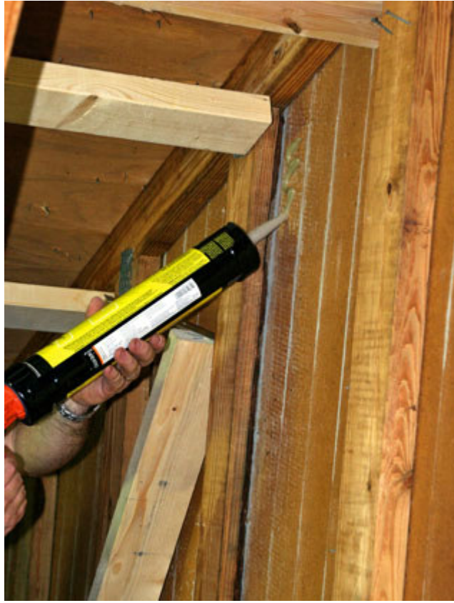
Figure 19. Applying construction adhesive where retrofit stud will make contact with the sheathing
